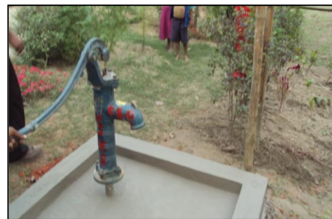
A view of new hand pump installed under the programme for augmentation of drinking water supply in villages in Bihar
